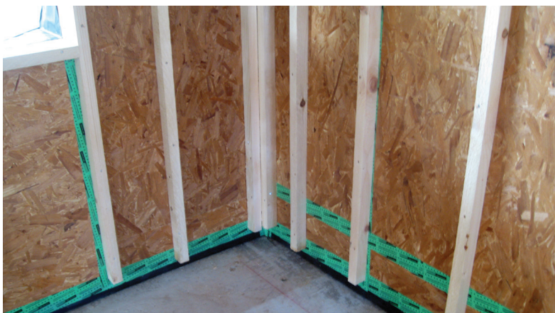
ABOVE: 18mm OSB-3 with joints taped successfully installed as airtight membrane. Photo: Eco Arc Architects
