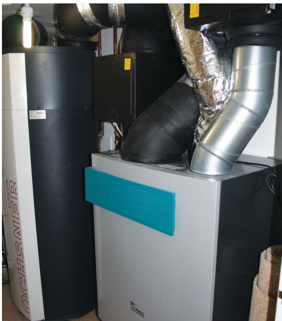
MVHR with heat pump in small services room Photo: Kirsty Maguire Architects
