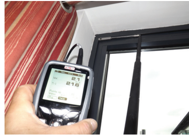
Extending vane anemometer showing a high air velocity of 2.1m/s through a gap at the head of a balcony window
