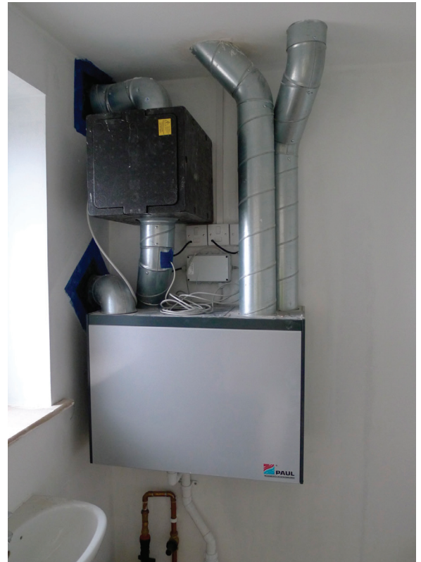
Paul MVHR Unit with optimised duct lengths (pre-insulation). Photo: Alan Clarke
