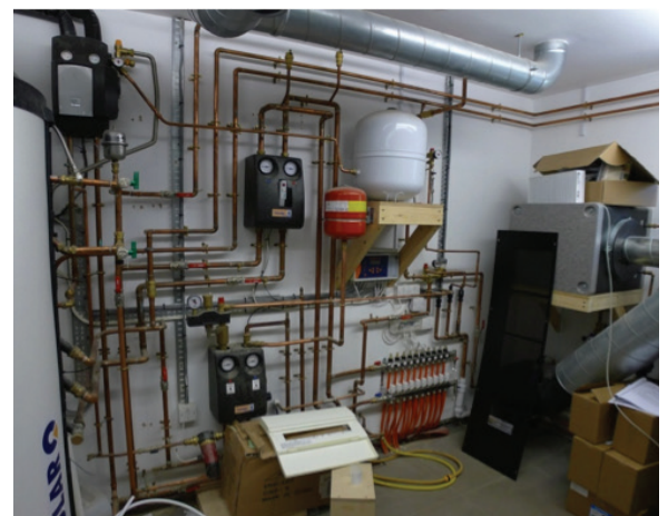
An unfinished plant room. Photo: Nick Grant
