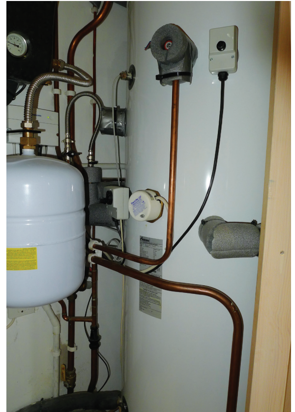
ABOVE: Water tank located in a cupboard. Photo: Alan Clarke
