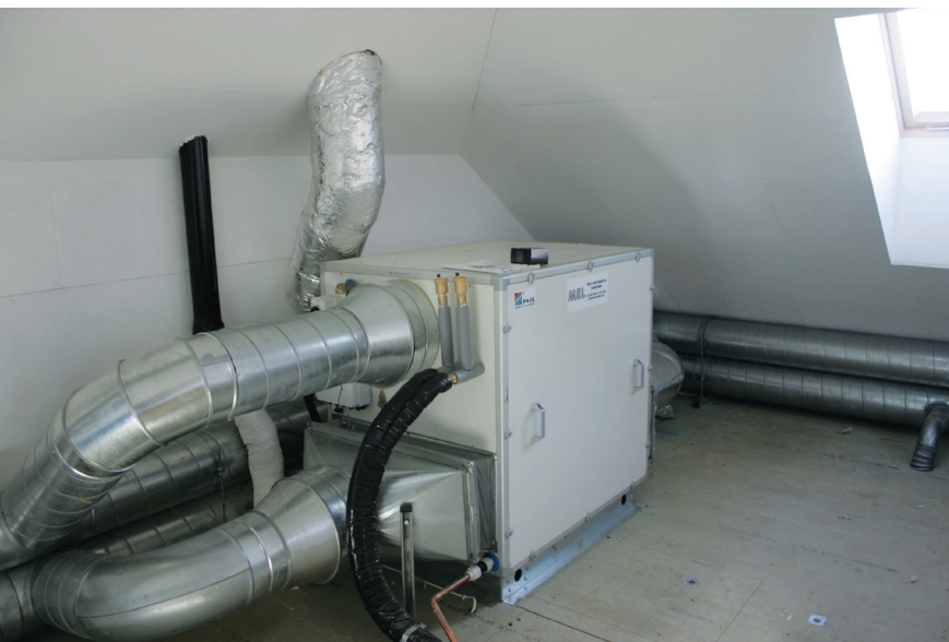
Large Paul MVHR unit. Photo: Conker Conservation
